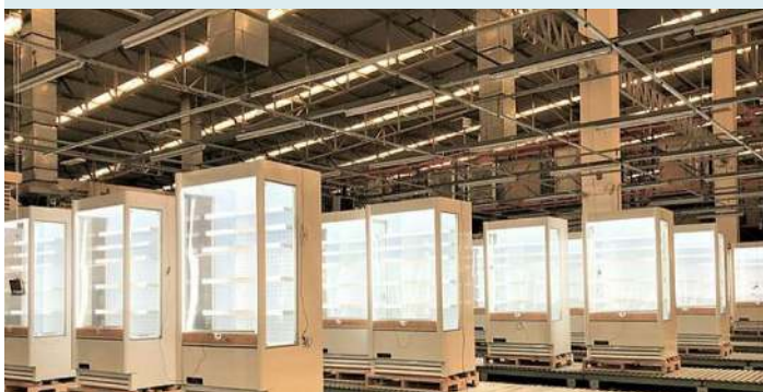
Green cooling technology in a warehouse. © GIZ Thailand
