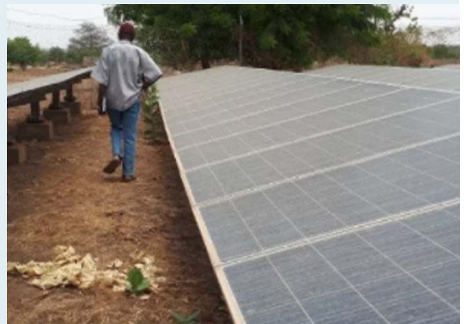
Individual walking past solar panels at facility © UNDP
